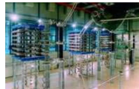
Power transmission infrastructure
