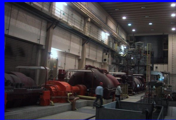
Huntorf, Germany, 290 MW
