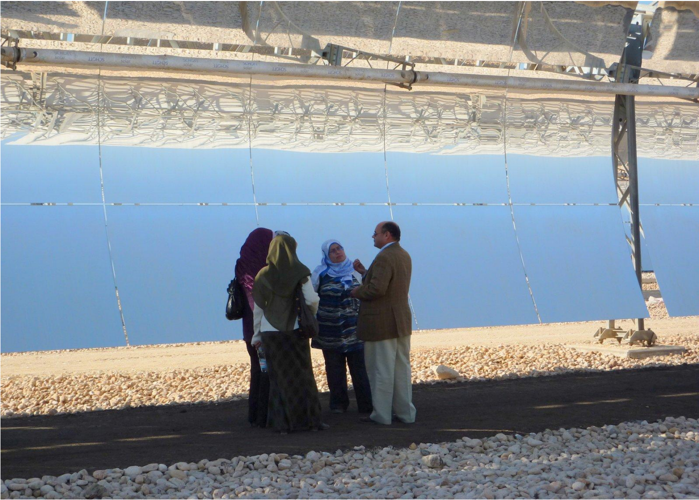
CSP solar plant at Kuraymat Egypt
