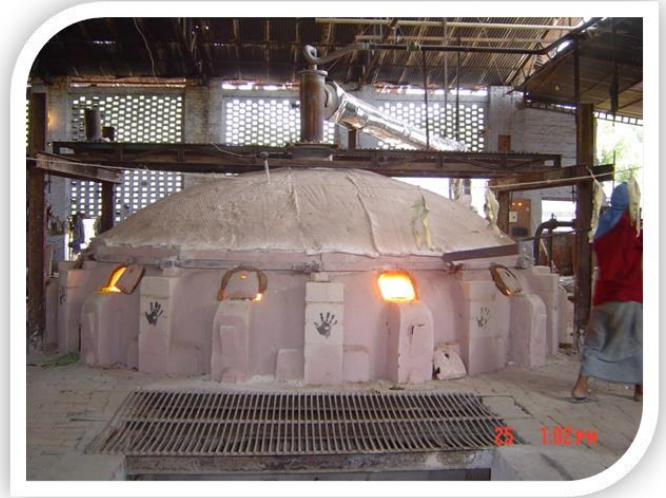
Recuperative natural gas fired pot furnace
