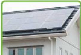
Solar panel (3.2 kW)
