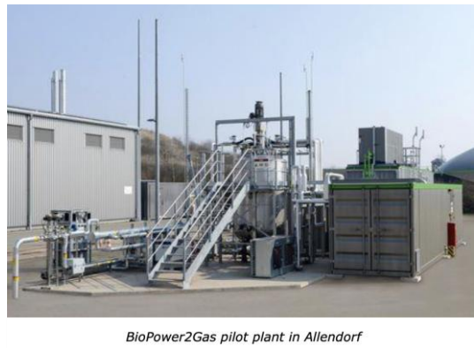
BioPower2Gas pilot plant in Allendorf
