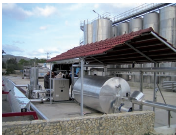
▲ A solar heating and cooling installation at a vineyard (Tunisia), one of 12 demonstration projects monitored under the SHC IA.
