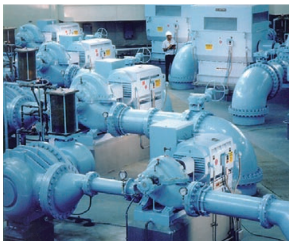
▲ Downsizing and using variable frequency drive for partial load reduce annual electricity use of 50 kW pump motors by 50%.
