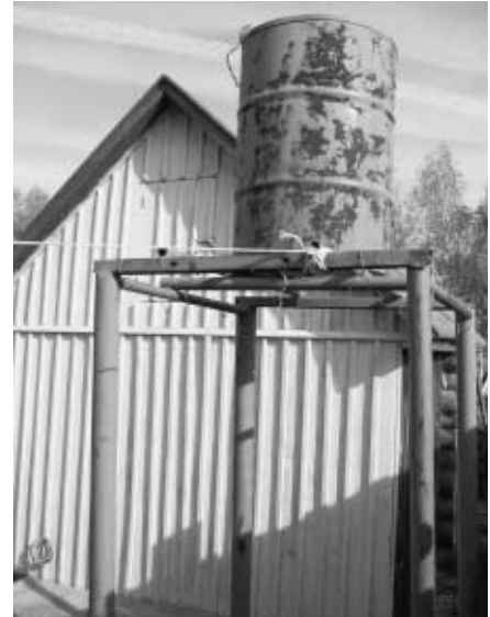
Figure 11 Primitive Solar Water Heater
