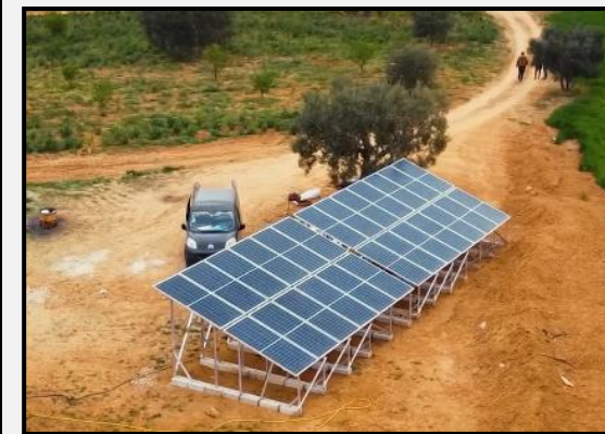
10 kWp solar PV pumping system in Chorbane, Tunisia
