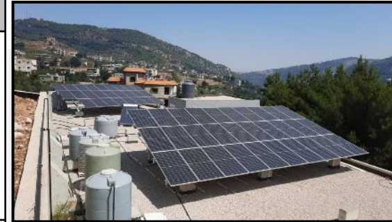
25 kWp solar PV system and solar water hearing system in Akkar, Lebanon
