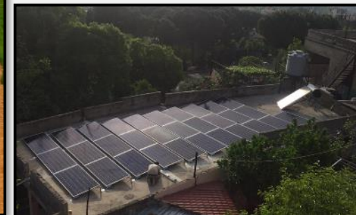
10 kWp solar PV system in Akkar, Lebanon
