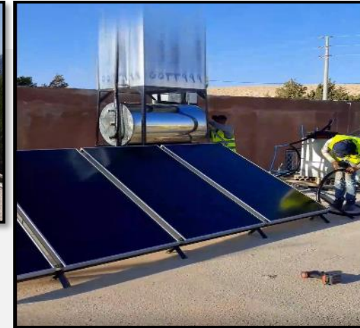
Solar water heating system in Maan
